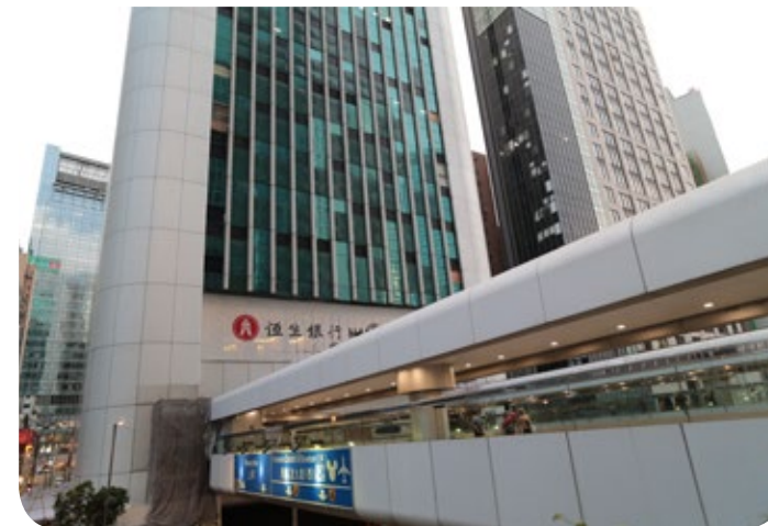
圖二：中環商業大廈的玻璃幕牆損毀情況(岑智明攝) Figure 2: Damages of glass curtain walls of Central commercial buildings (courtesy of Shun Chi-ming)
